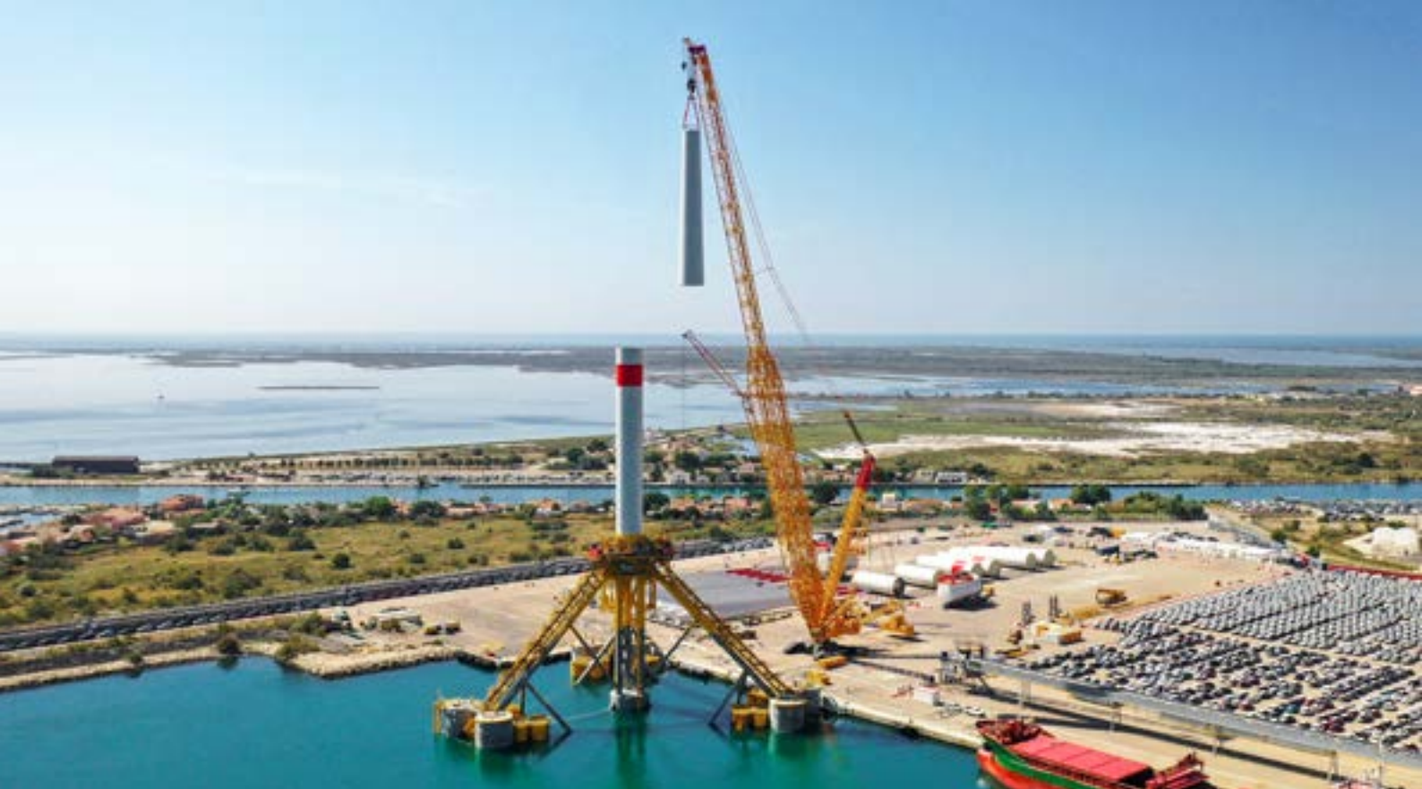
A Liebherr LR 11350 crawler crane is installing three 8.4-megawatt wind turbines on floating platforms in the harbour of Port-Saint-Louis-du-Rhône. Foto: Iann Hanning
