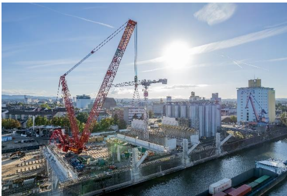
liebherr-lr-11000-egger-4.jpg The LR 11000 moves a girder with a gross weight of 211 tonnes over a 59-metre radius.
